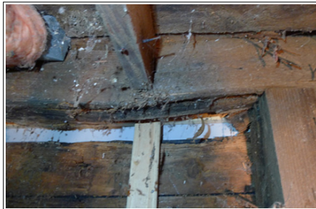
The mud sill from inside, under the house. Note the deflection in the beam to the left of the floor joist, just right of the pink insulation on a heat duct.
